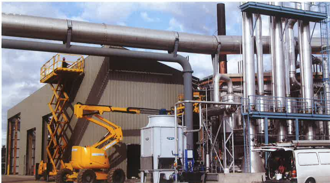
The finishing touches are being made to the building in front of the tripple effect 'waste heat evaporator' system
