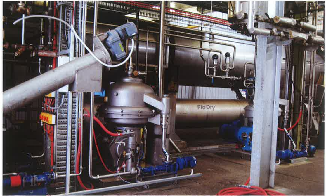
The heart of the plant... the rotary Flo Dry dryer can be seen in the background and one of the new G Tech separators is in the foreground.
